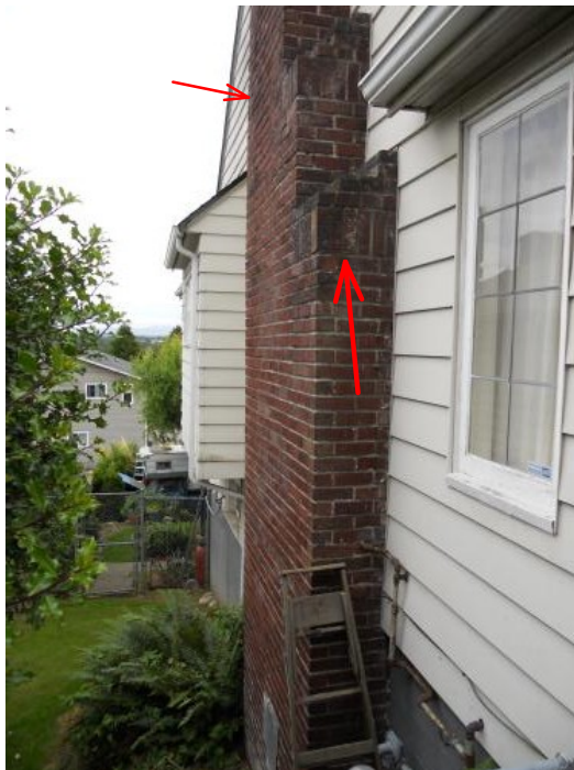
#7 Chimney in need of maintenance/ re-pointing of mortar joints.
