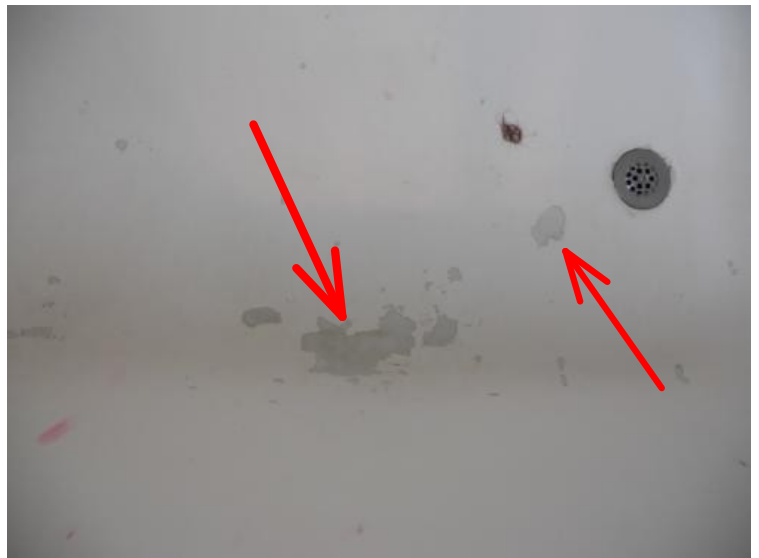
#24 Tub in downstairs bath has peeling epoxy coating.
