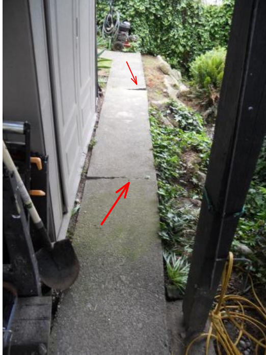
#5 Settling and trip hazard cracks in walkways.
