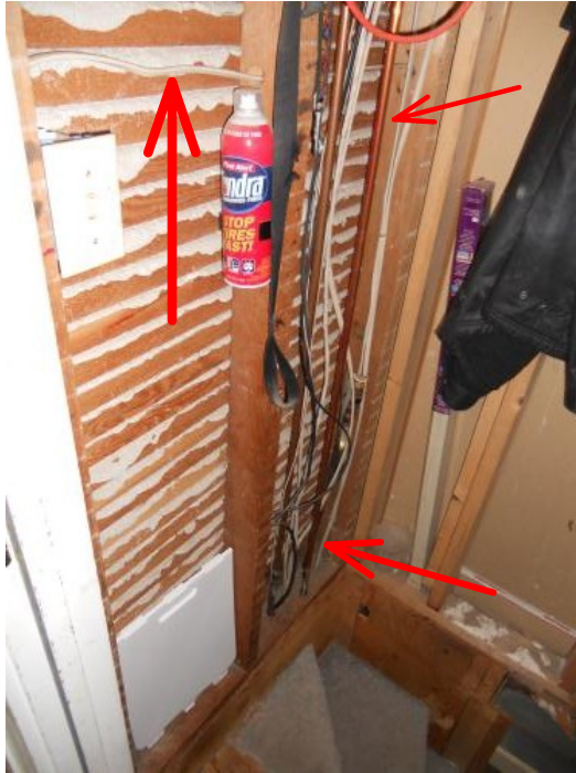
#25 Unfinished walls in basement stairwell have exposed wiring and plumbing.
