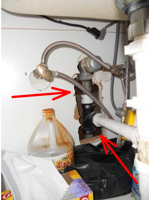
#29 Open wall where plumbing enters under kitchen sink should be sealed off.
