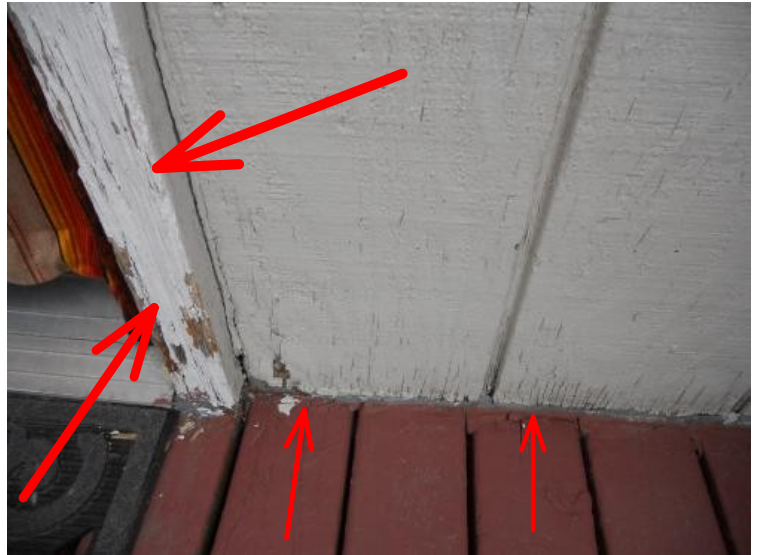
#30 Wood in need of repair at entry to deck from kitchen/dining room. Decking is not properly flashed at siding junction and in need of caulking.
