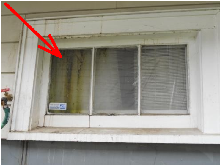
#9 Signs of leak from inside basement plumbing.
