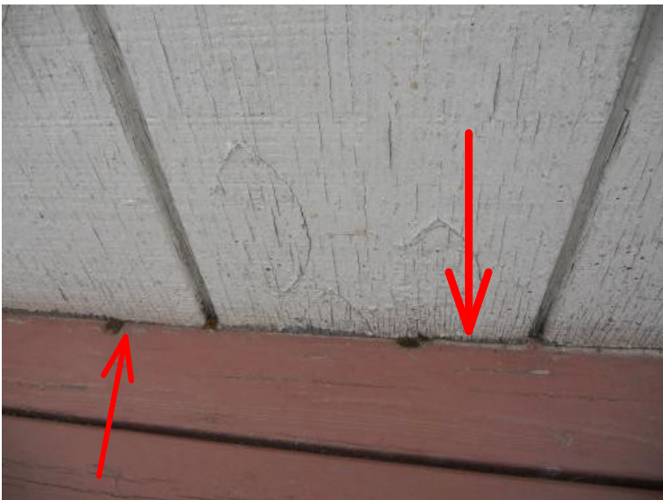
#31 Decking is not properly flashed at siding junction and in need of caulking.
