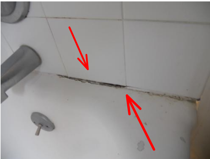
#23 Caulk needs replacement/repair in downstairs bath.
