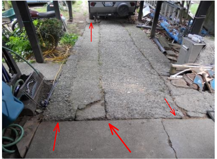
#6 Settling and trip hazard cracks in walkway/ driveaway.
