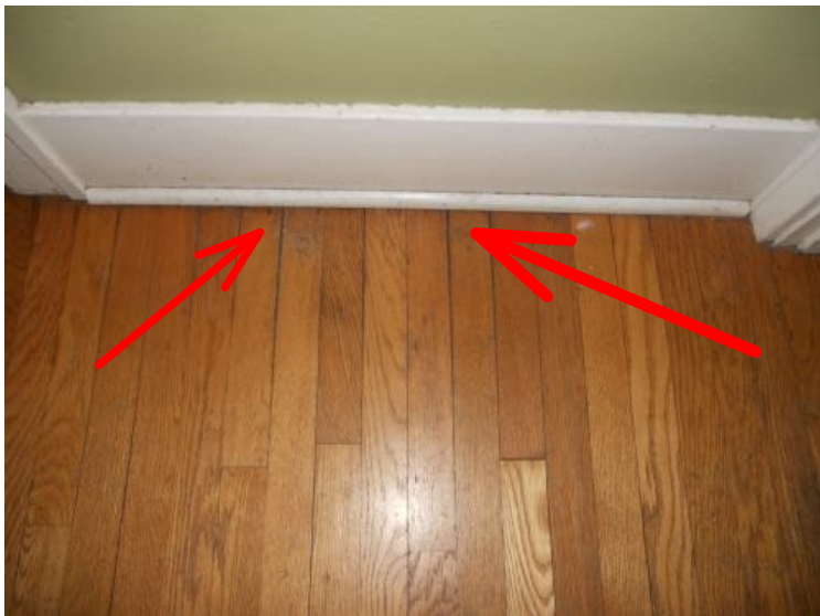
#27 Open gaps and in need of refinishing noted in main level hardwood flooring.
