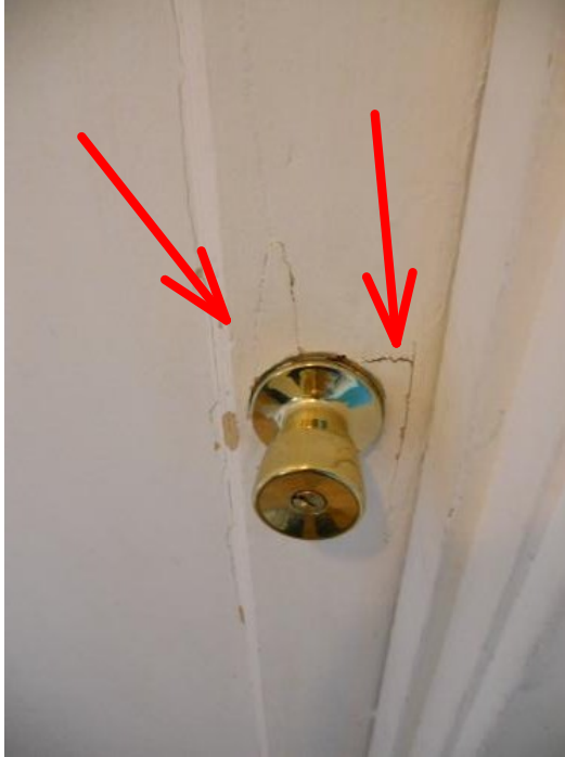
#21 Structural cracks in east bedroom door.
