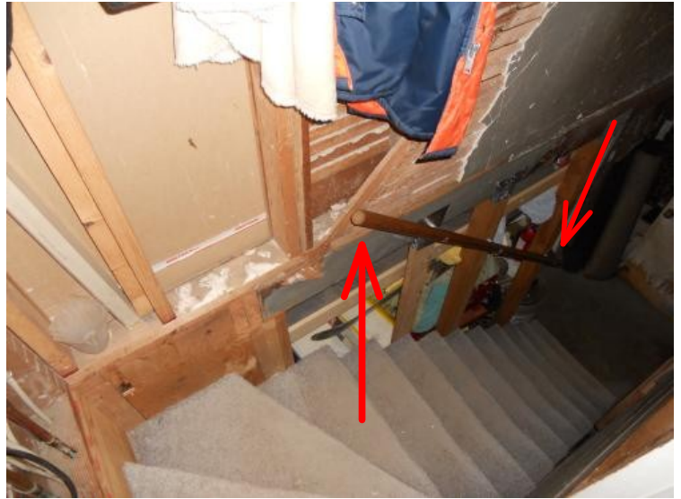
#26 Handrails do not extend entire length of stairwells.
