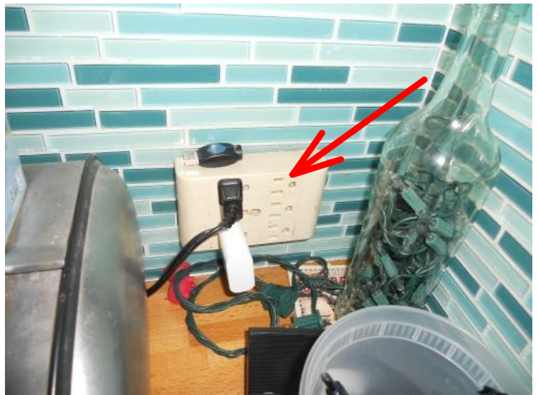
#20 Non GFCI outlet near kitchen sink.
