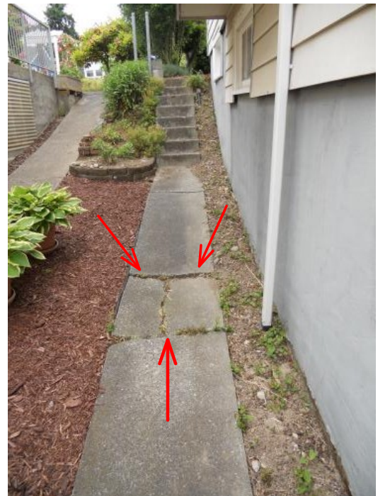
#4 Settling and trip hazard cracks in walkways.
