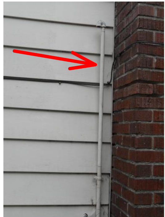
#8 Sign of underground oil tank.
